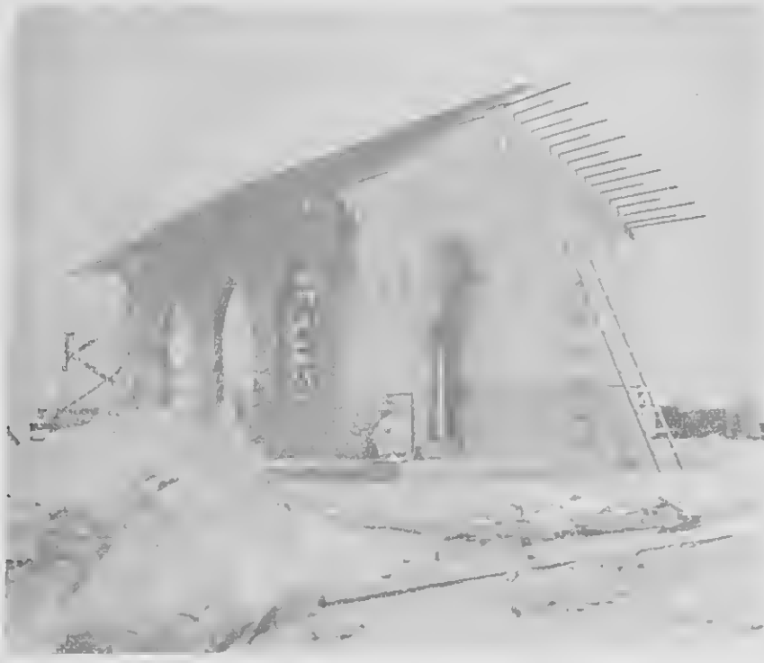
NEW CHAPEL: As the construction of the new chapel at Alto Vista nears completion, white quartz crystals are inlaid into the walls which will form, in the bright Aruba sunshine, a sparkling halo around the chapel's base. CAPILLA NOBO: Mientras construcción di e capilla nobo na Alto Vista ta acercando completacion, piedra di cristal ta wordé poni den e mureta cual lo forña, den e claridad di solo heñante na Aruba, na cielo iluminoso rond di base di e capilla.
